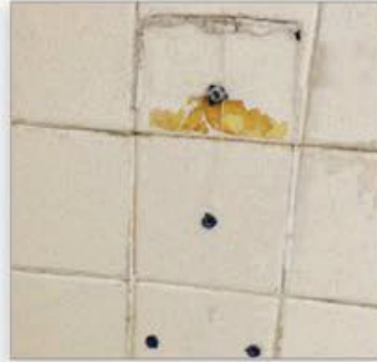
RIPPED OFF THE WALL
